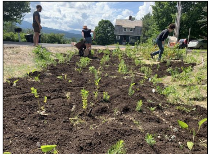
Bioretention Raingarden in Hyde Park
