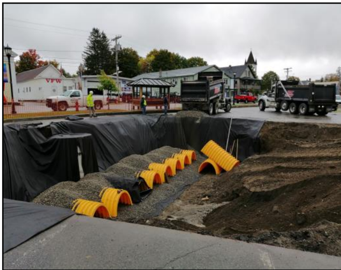
Sub Surface Infiltration Chambers in Morristown
