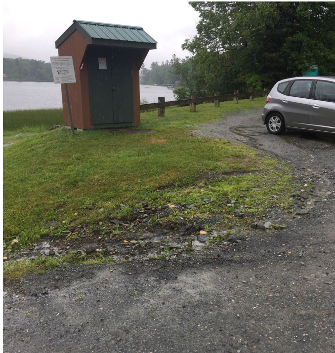
Figure 7: Erosion at the VT Fish and Wildlife Boat access observed during a storm event in June 2019. The concept design for this area (SW-4) describes a BMP that would treat this runoff.
