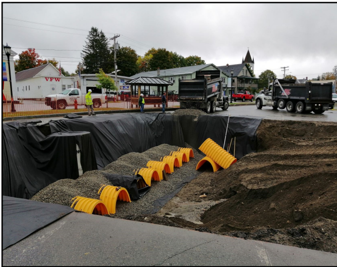
Sub Surface Infiltration Chambers in Morristown
